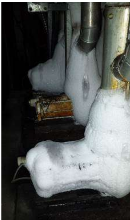
3 pompes Hermetic Pumpen BmbH
